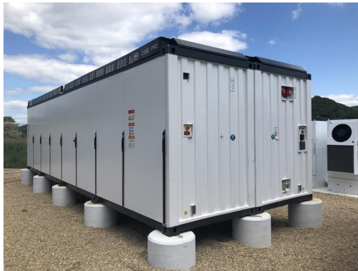
Alliant Energy's battery storage system in Boaz, Wisconsin
